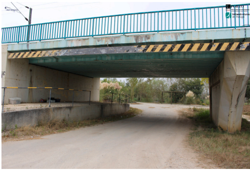
Fig. 8. Canelas bridge. (a) cross-section (unit: m) (adapted from Pimentel et al. [41]); (b) view of the first span.
