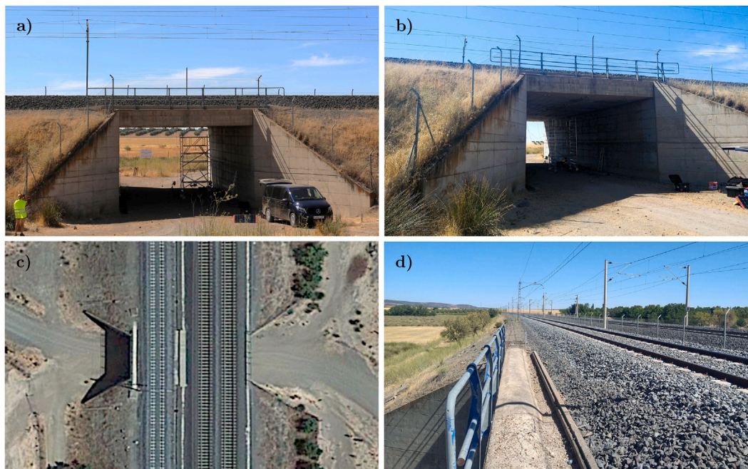
Fig. 1. Images of the underpass under study: (a–b) the bridge, seen from the HS side, (c) a satellite image of the structure [22], and (d) a view of the bridge deck next to the conventional track.
