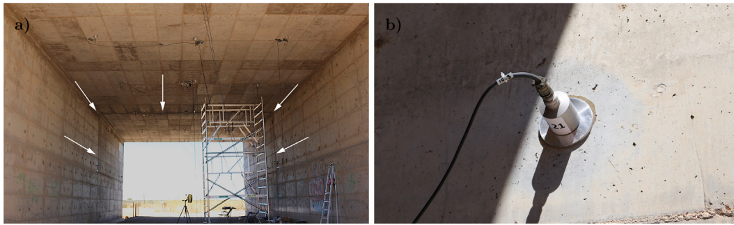
Fig. 2. Bridge setup during the experimental campaign: (a) sensors on the slab, where the white arrows mark the position of the longitudinal joint, and (b) an accelerometer installed at the bridge wall. (For interpretation of the references to colour in this figure legend, the reader is referred to the web version of this article.)
